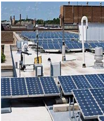
Common PV system installation practices expose your roof to severe windstorm damage
