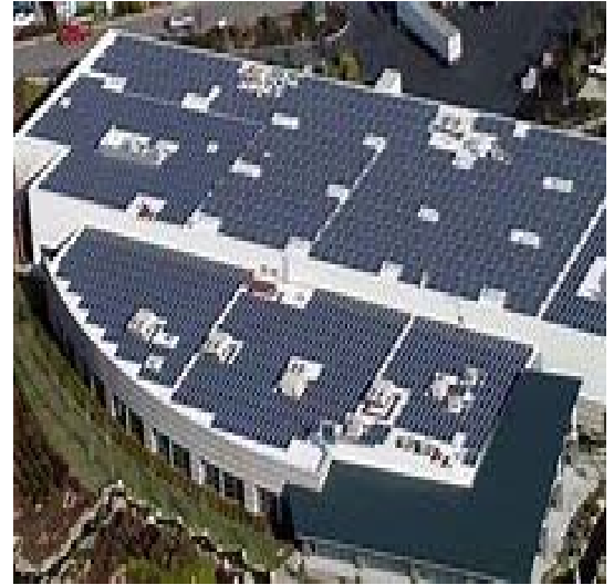
Typical rooftop PV system with panels near the roof edges
